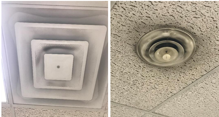
Several types of typical supply diffusers
