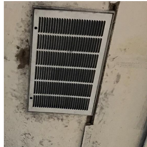
Typical return grille
